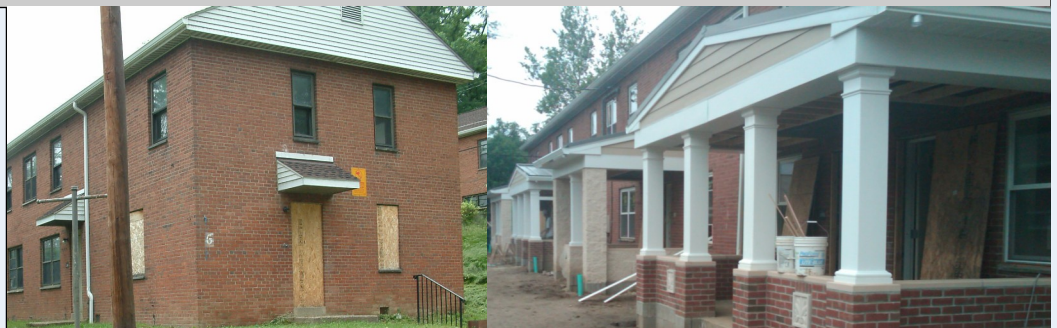
William H. Day Homes Before and After The Harrisburg Housing Authority anticipates completing the renovation in the next few weeks.
